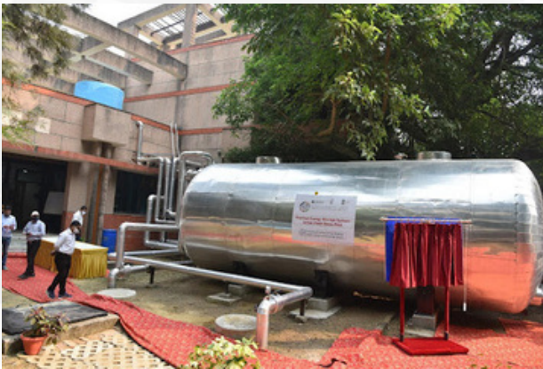
Figure 9: Thermal Energy Storage System Horizontal Outside Tank
