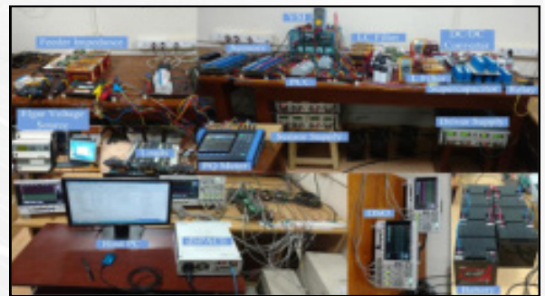
Figure 69: An integrated microgrid system with various renewable energy sources and storage units
